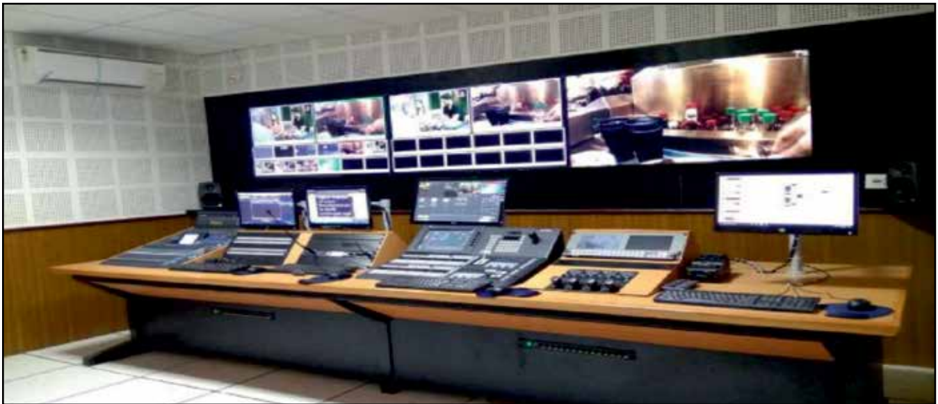
Production Control Room
