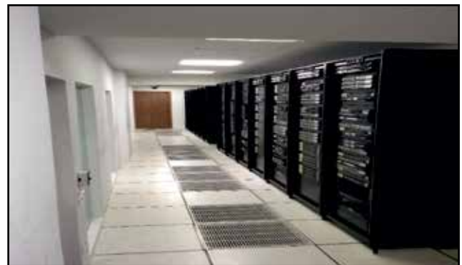
Data Center: Itanagar
