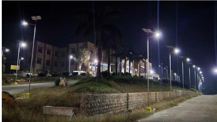
SITC of LED Street Lights and High Mast Lights at College of Horticulture of Koppal
