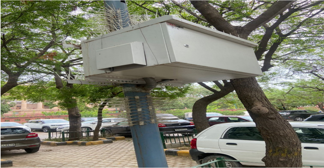
Insulated Rack for power supply to Cameras for any type of weather-CCTV System of MHA
