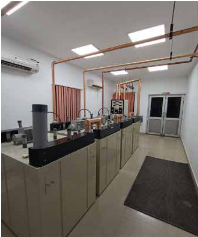
CTI Coimbatore Combiner Room
