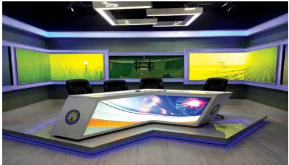
Supply, Installation, Testing and Commissioning of MOOC TV studio at Indira Gandhi Krishi Vishwavidyalaya, Raipur
