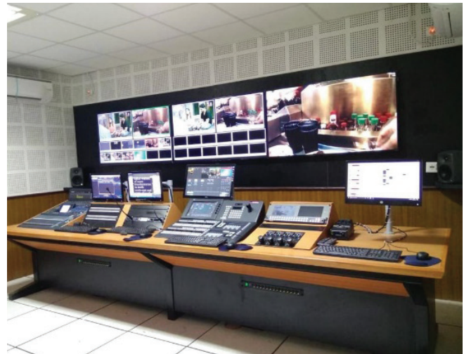
Supply, Installation, Testing and Commissioning of Studio Broadcast Equipments along with Infrastructure works for Visva-Bharati
