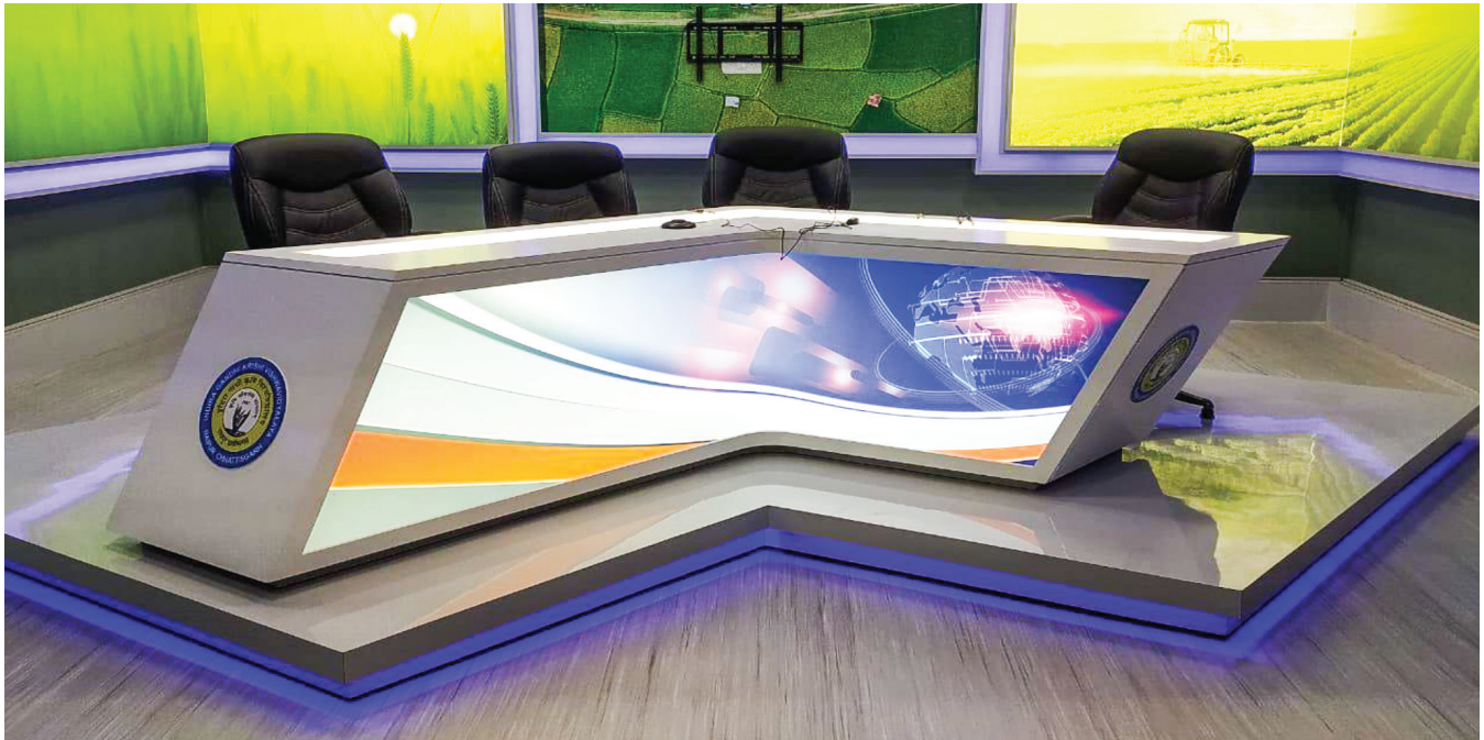
(Setting up TV Studio with related acoustics and electrical works for the preparation of MOOC's at Indira Gandhi Krishi Vishwavidyalaya (IGKV), Raipur, Chhattisgarh)
