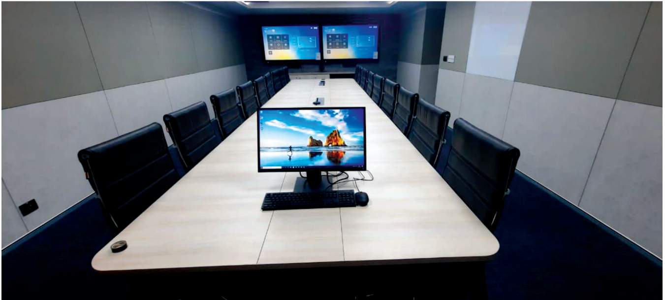
(Setting up of multiple facilities viz. Video conferencing, e-classrooms for the digital academy and center for PSS in disaster management in new building at NIMHANS, Bangalore)
