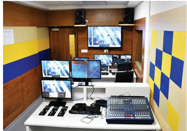
Production Control Room
