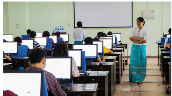
Supply, Installation, Testing, Commissioning and Onsite support for classroom equipment for Myanmar Institute of Information Technology at Mandalay, Myanmar.
