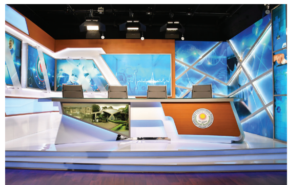
Setting up of HD TV studio, IR studio and Digital Signage systems for JIPMER, Pondicherry
