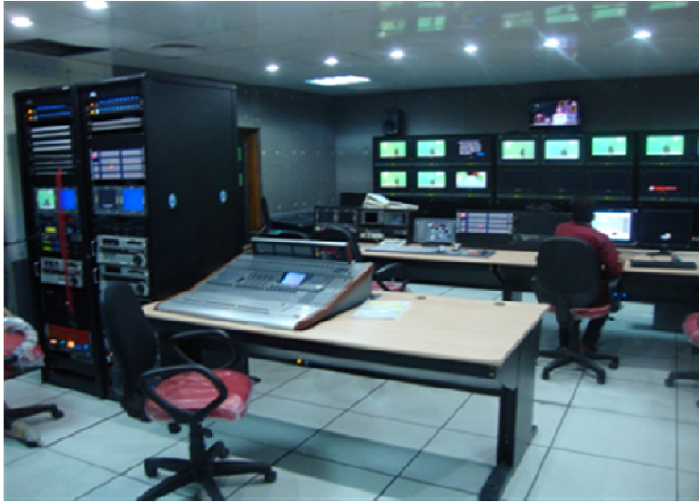
A view of News Studio at Bangladesh TV completed and handed over by BECIL
